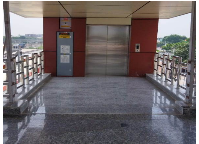
Lift at BSBS station
