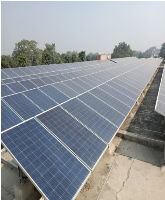
Solar Panels at DRM office Varanasi
