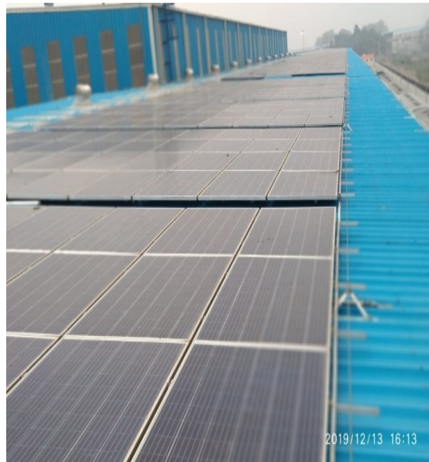
Solar Plant at DEMU Shed ARJ
