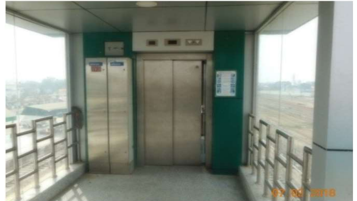
Lift at MUV
