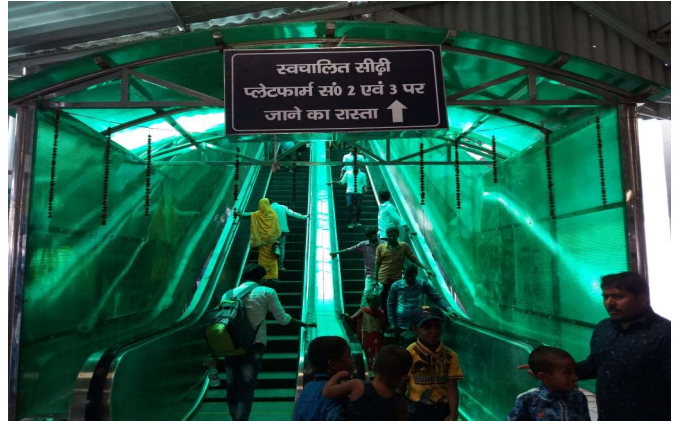
Escalator at MUV Station
