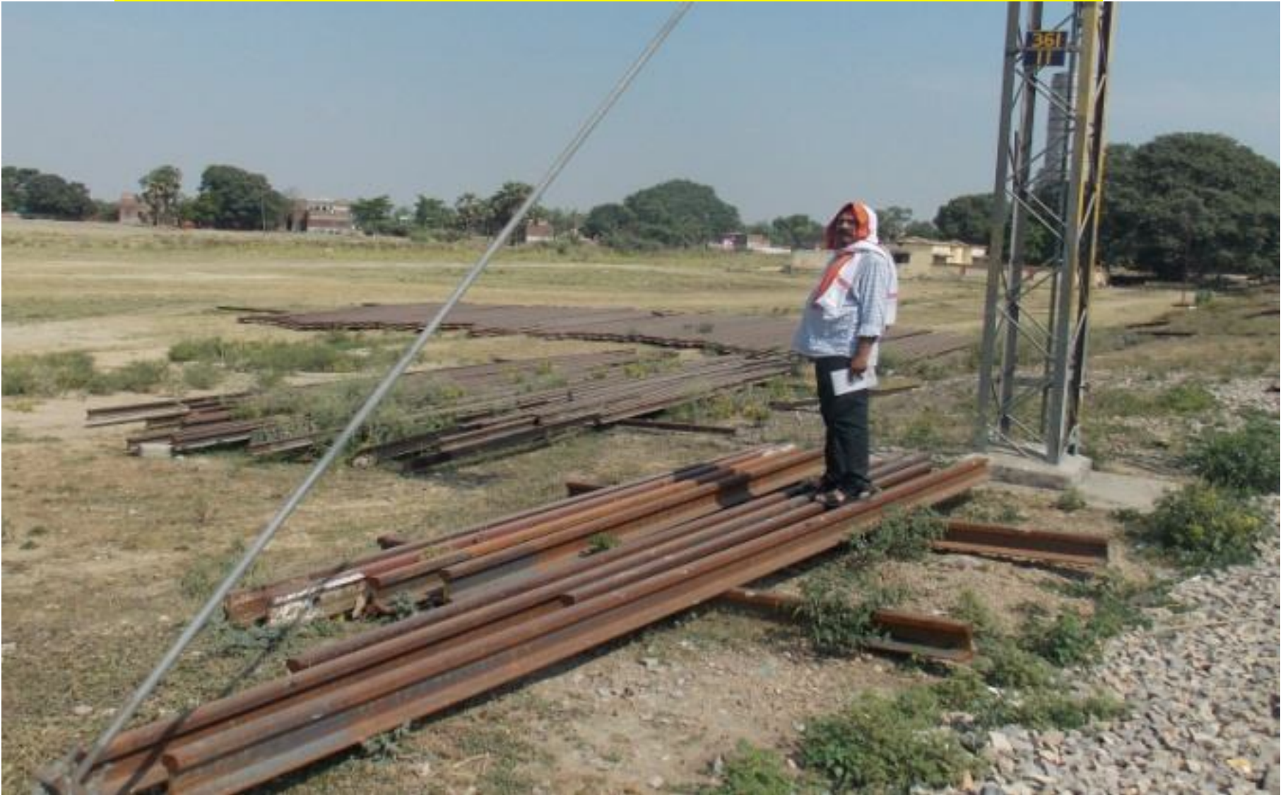
Location RE Pole No.361/11, 10MT Apx., 52KG Rail
