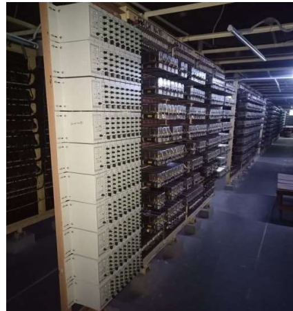
Relay Room at Gorakhpur Station
