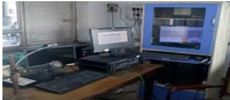
Public Address System at Mau Jn.
