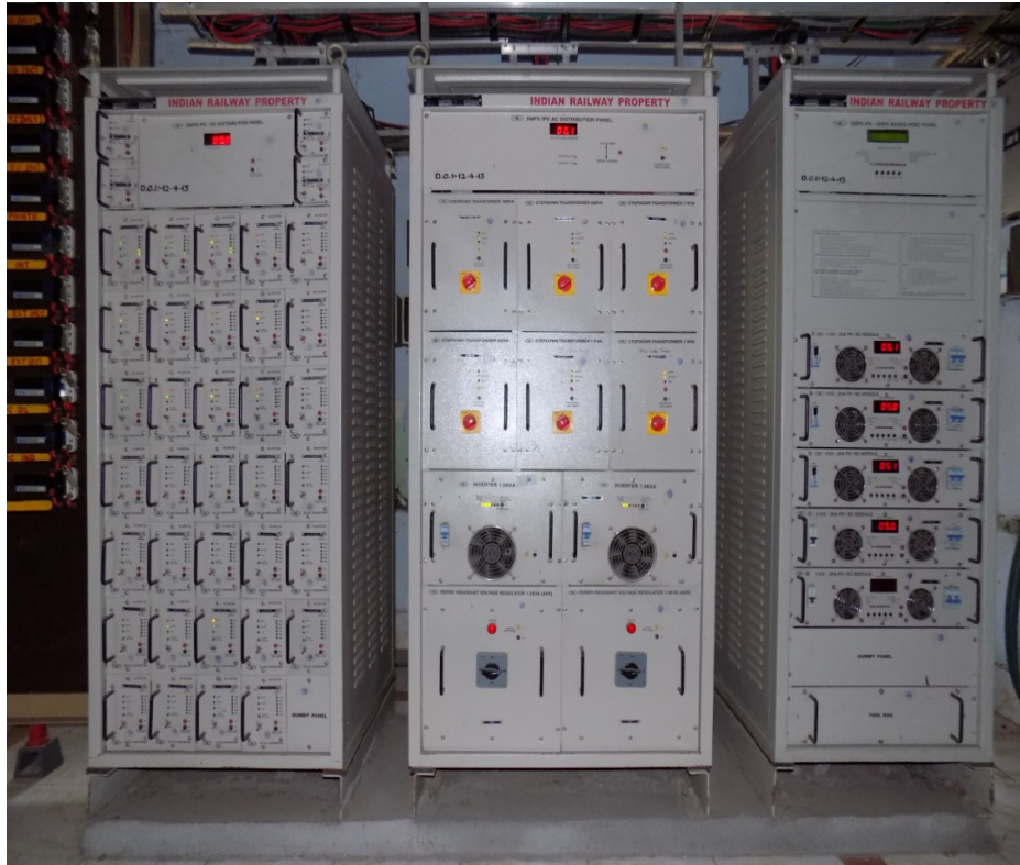
Intergrated Power Supply (IPS)
