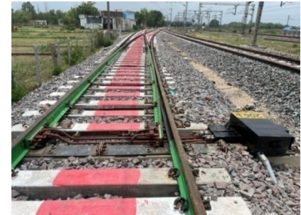
Electric Point Machine
