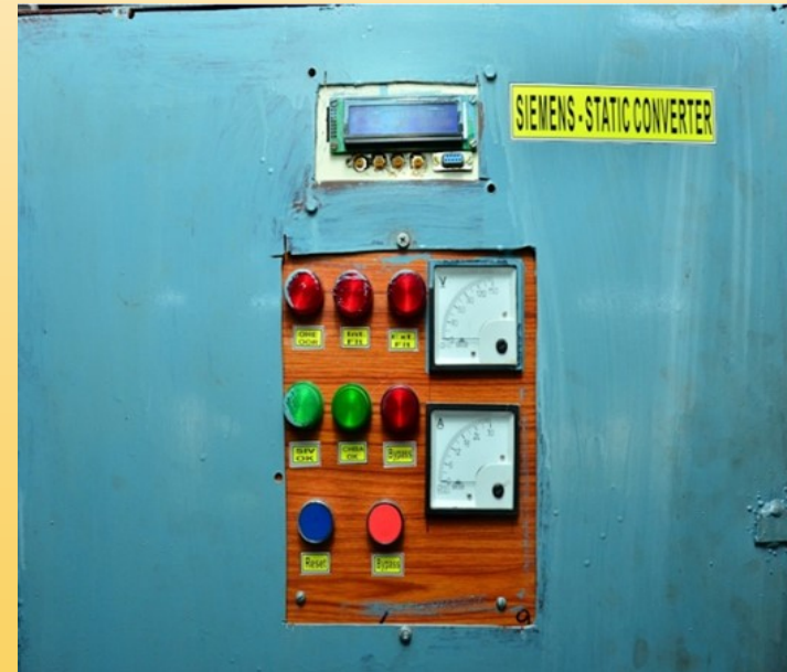
Static Inverter Panel for Displaying and mode of operation
