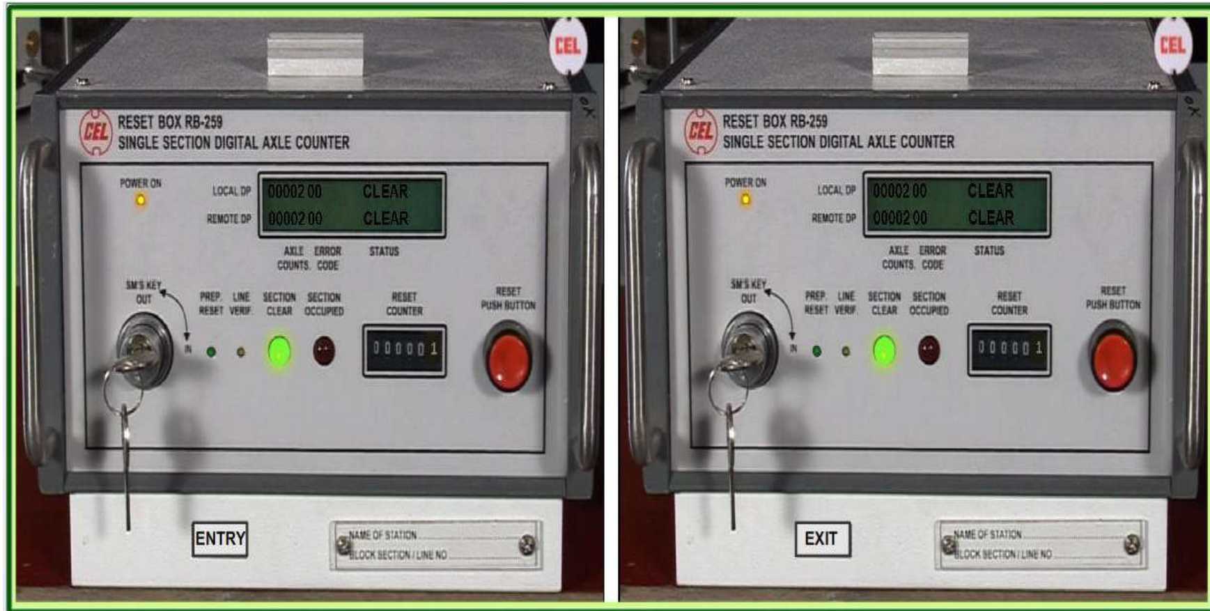
Reset box at ENTRY END & EXIT END
